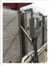
Variable Refrigerant Flow HVAC
