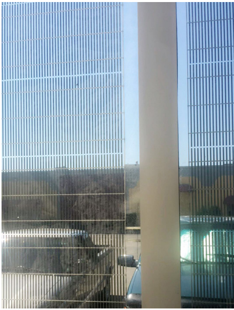
View through PV curtain wall
