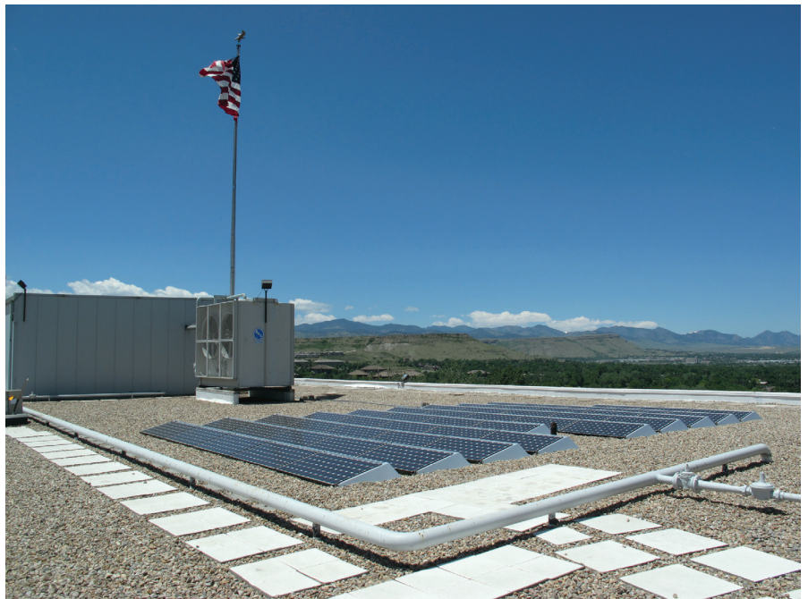
An Indirect/Direct Evaporative Cooling unit installed at Golden Hill Office Center, Lakewood, CO (Source: High Performance Buildings magazine)
