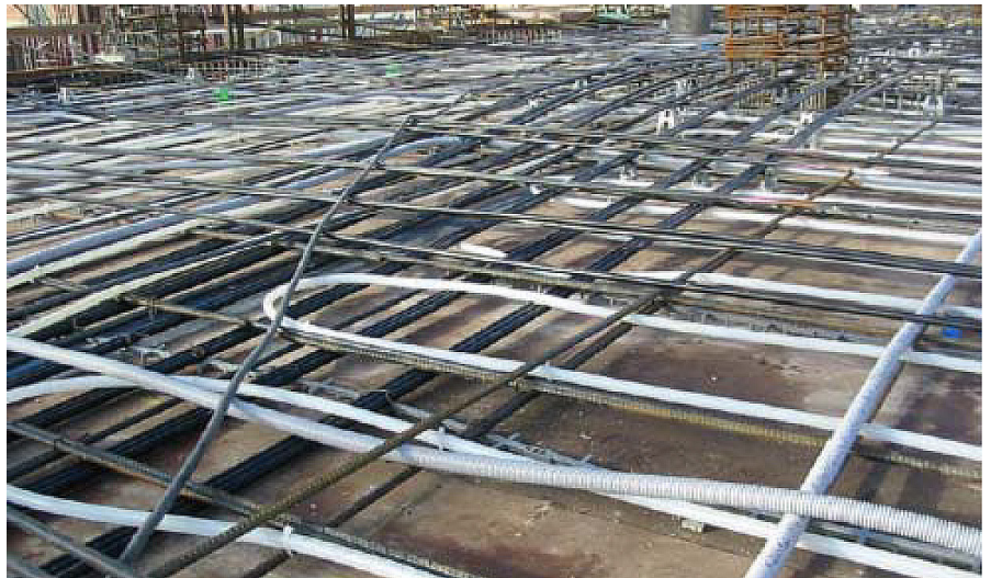
Radiant piping system at David Brower Building (Courtesy: High Performance Buildings magazine)
